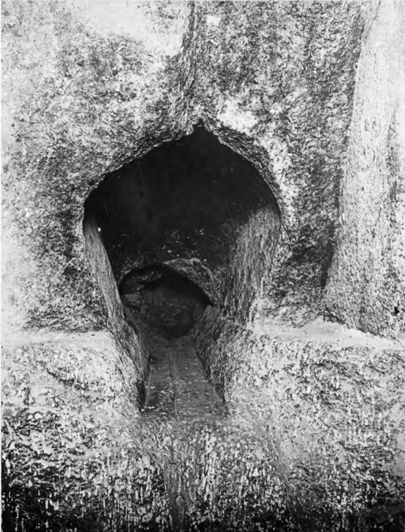
The mouth of the air-channel in the south wall of the King's Chamber
